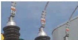
TRANSFORMER INCOMING AND OUTGOING LINE
